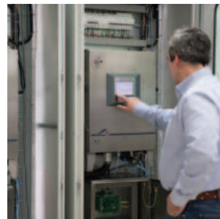
GAS ABATEMENT MONITORING OF MULTIPLE GASES
