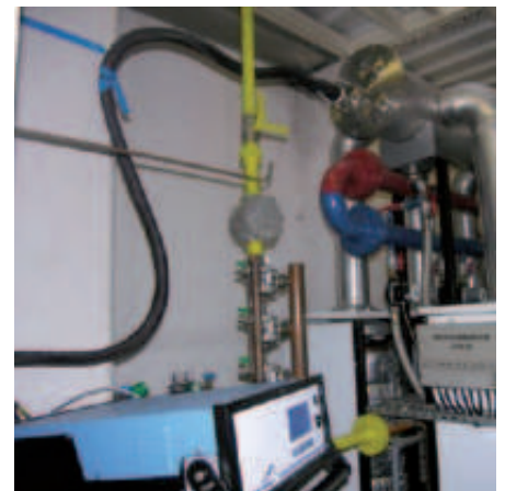
MONITORING OF COMBUSTION GASES ON INDUSTRIAL FURNACE
