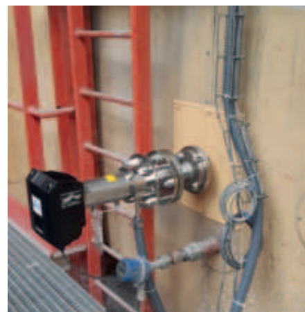
CROSS DUCT, INLINE COMBUSTION MONITORING
