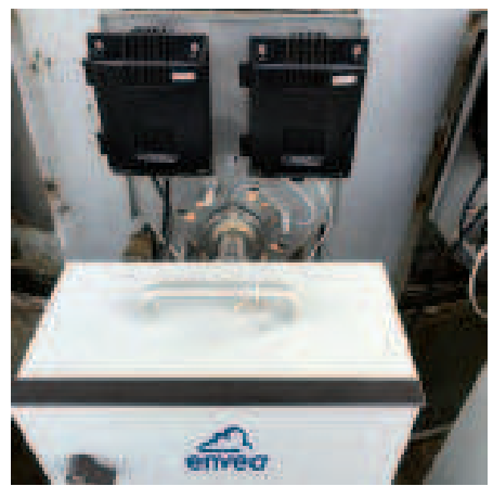
STACK OR DUCT ONLINE MONITORING
