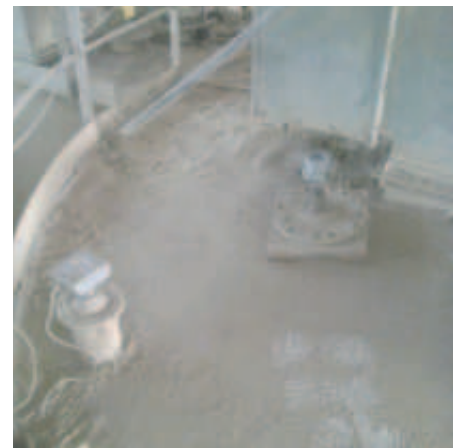
INSTALLATION FOR LEVEL MEASUREMENT IN SILOS
