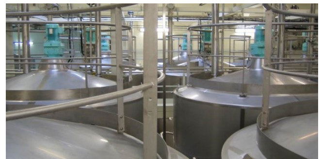
Figure 5: Alternatively, raw milk storage tanks can be installed indoors.
