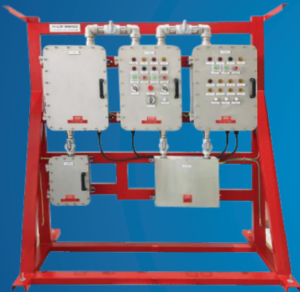
FOAM GENERATOR CONTROL SYSTEM
