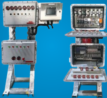
CHEMICAL INJECTION SKID CONTROL SYSTEM
