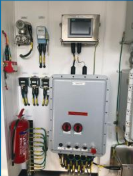
PLC BASED HVAC CONTROL SYSTEM
