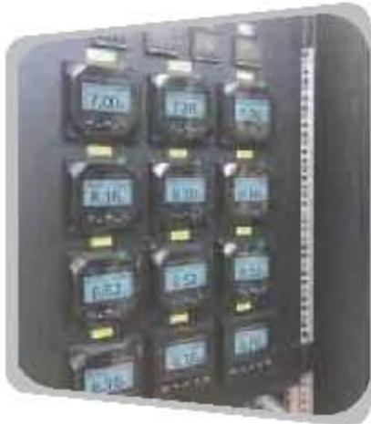
pH controller EC controller
